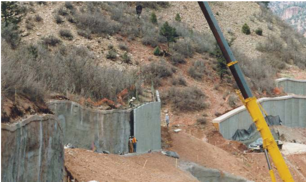
Figure 1. Photo. Installation of a permanent pre-cast concrete facing over a structural shotcrete soil wall.
